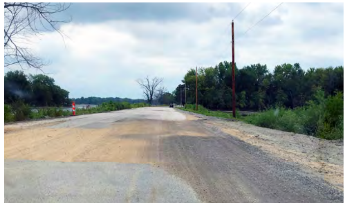
Entry Road covered in Sand
