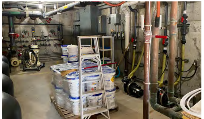
Storage within Equipment Room
