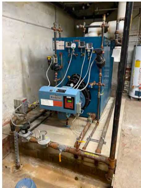
Utilities in Basement
