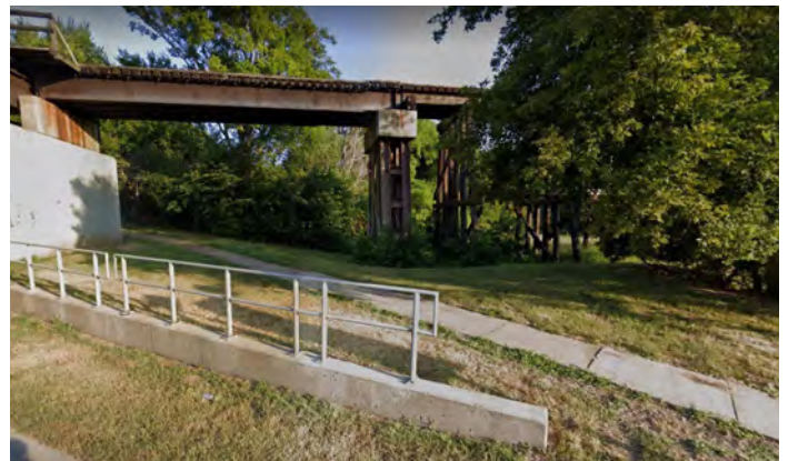
Sidewalk under Railroad Tracks PARKS CONDITION ASSESSMENT
