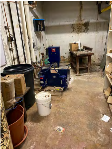
Utilities in Basement
