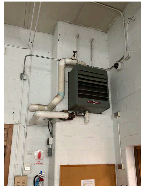
Utilities in Classroom
