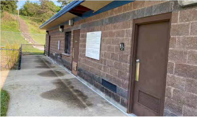
Restroom and Shower Facilities
